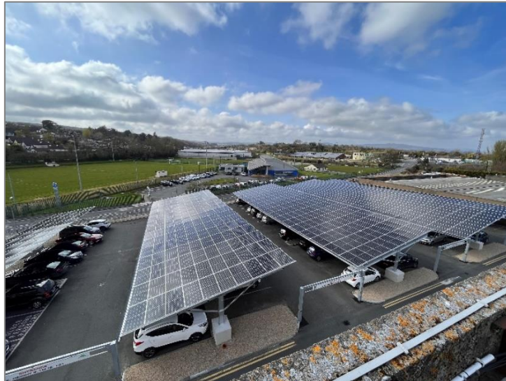
Figure 3.10: The solar panel covered car park facility in Wicklow that provides 300kW of renewable energy.
